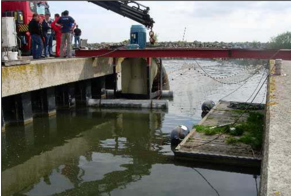
Figure 3.3 - View of the pump in the cage
